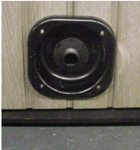
Figure 12. Cabinet mounted drain valve
